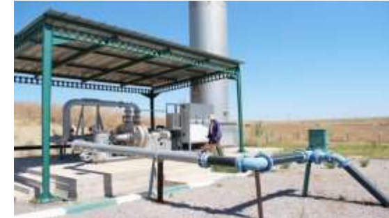
WASTE TO ENERGY
