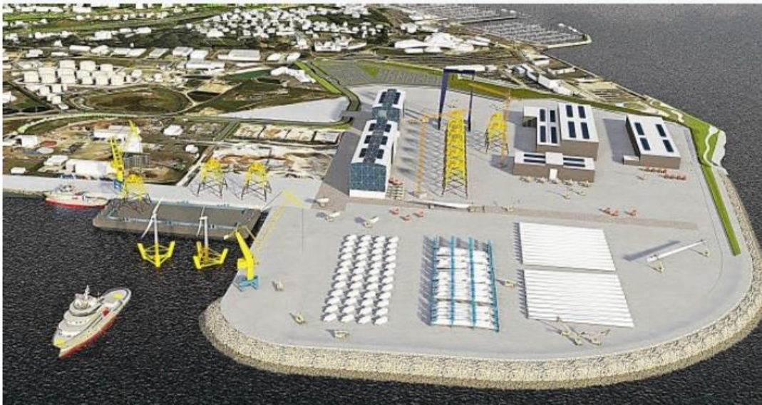
Work in progress for the construction of a polder in the port of Brest aimed at
